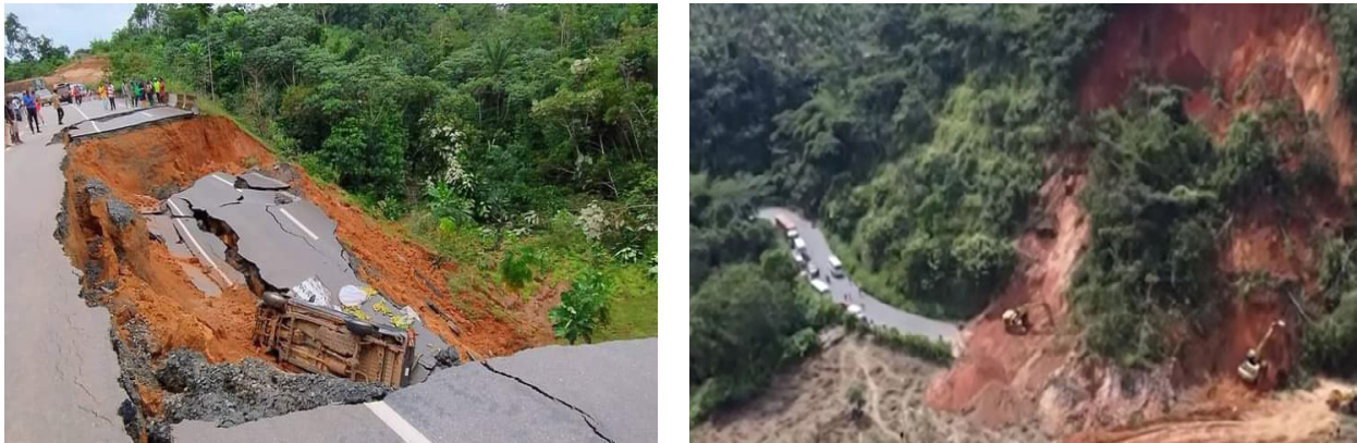
Figure 12: Extreme weather events and infrastructure deterioration (subsidence of the Bonepoupa-Yabassi highway (fig1) and landslide on the Dschang cliff(fig2)) source: www.cameroon-concord.com
