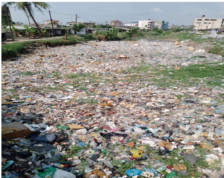
Overview of a drain blocked by plastic waste in Douala Bonaberi.
